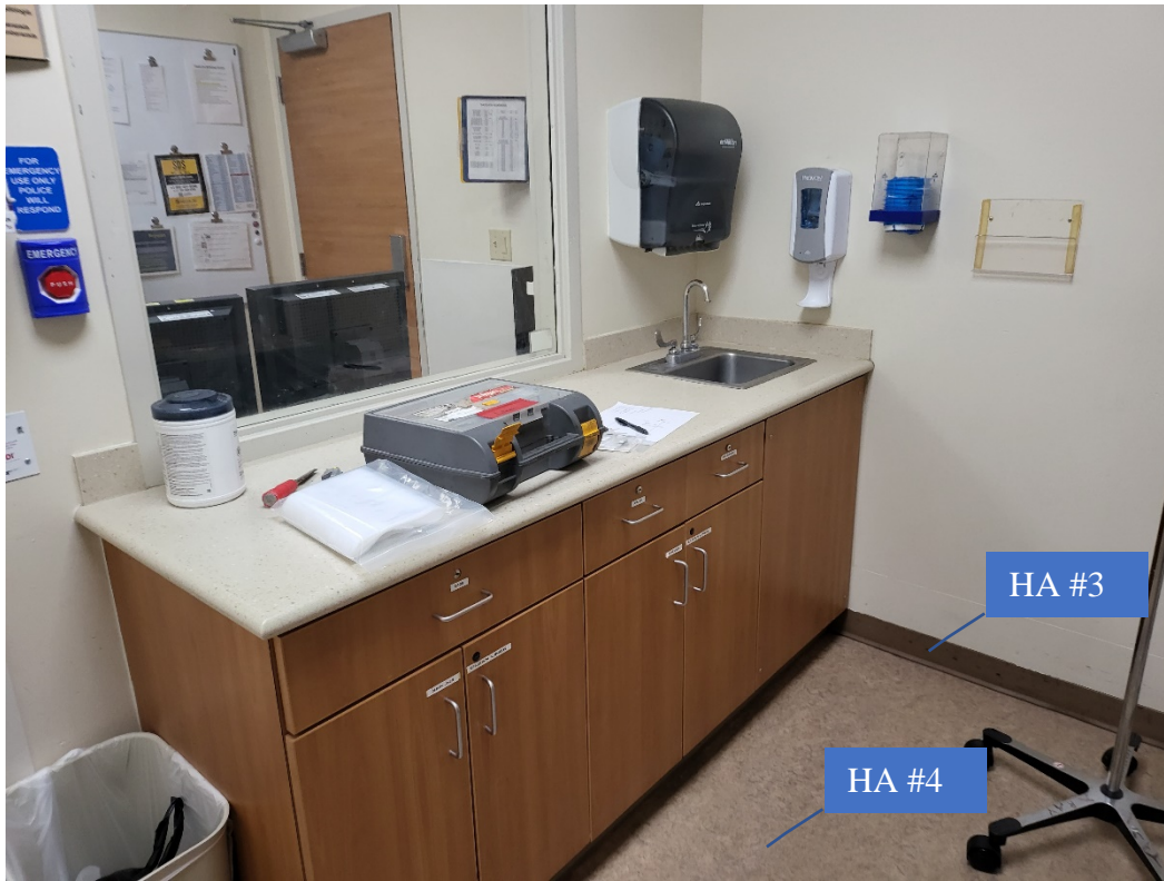
Photo 2: View of HA #3: non-ACBM 4" vinyl cove base (tan), & HA #4: non-ACBM sheet vinyl flooring.
